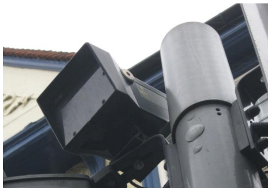
Figure 5.3: On-crossing detection unit
