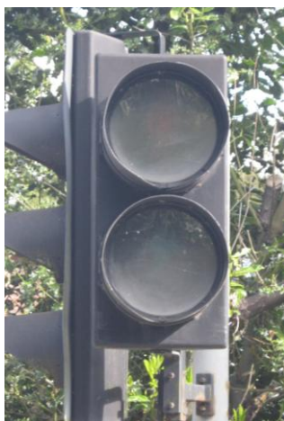
Figure 5.2: 'Blackout' at a farside pedestrian signal
