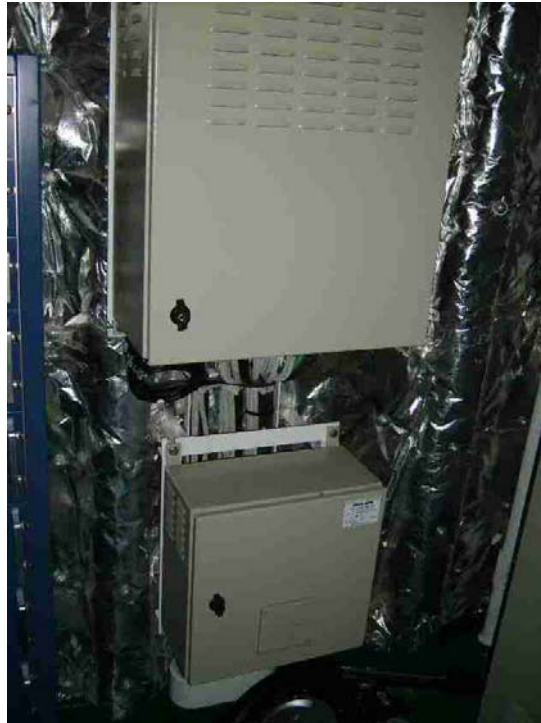
AVECS Room on the Bridge
