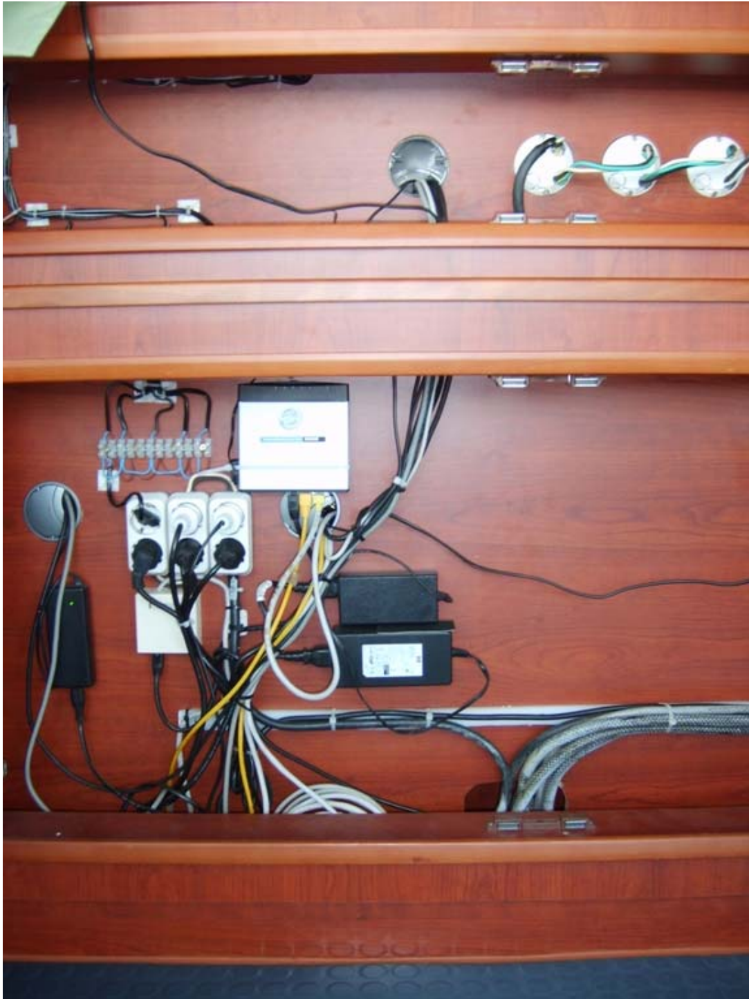
Siemens Linksys Switch in the backside of Bridge Computer office, no configuration needed
