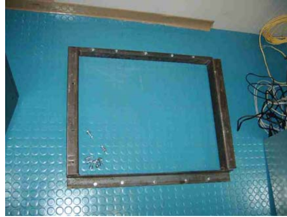
Foundation made of steel profiles welded, mounted and painted by the crew
