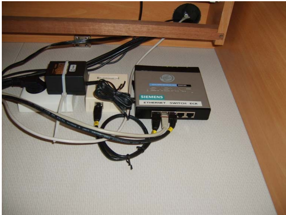
Siemens Linksys Switch in ECR, no configuration needed
