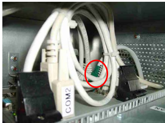
Spare cable for Chart Room connected
